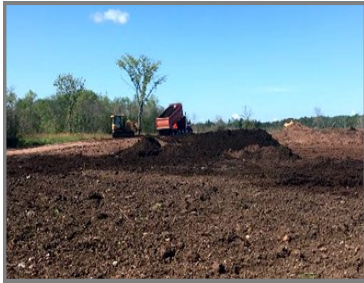
Locally-sourced fill, with a seed-bank of native species, was used to fill in the site.
