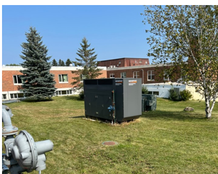
New generator to replace the previous unit.
