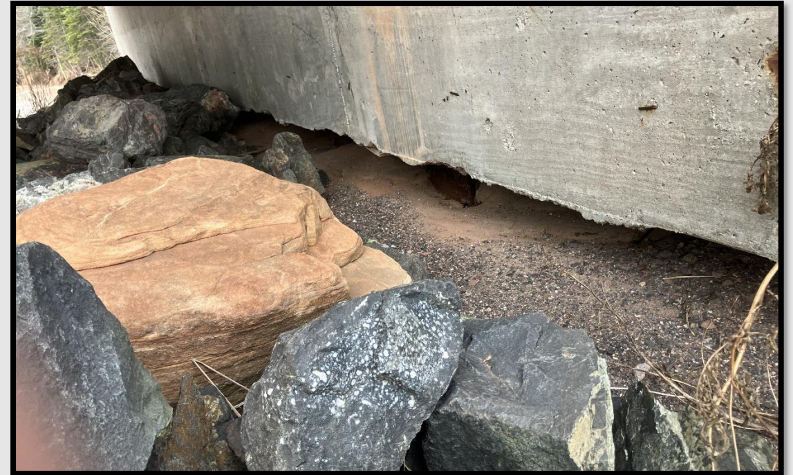
Settlement around Fish Creek Bridge abutment
